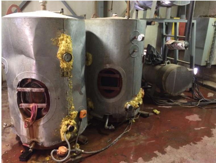
Old boiler system
